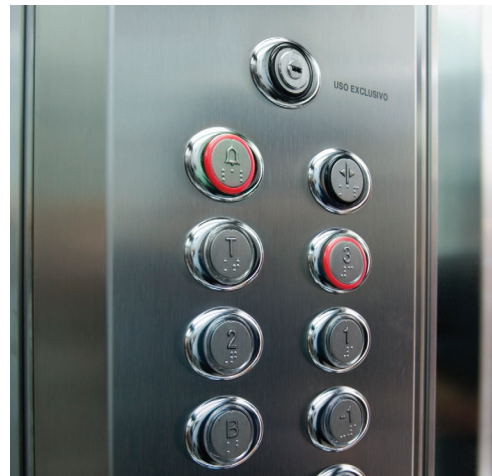
Elevator Controls Application
